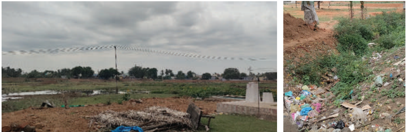
Figure 11 : Encroachments include illegal religious sites, fencing and drains blocked by silt and solid waste
